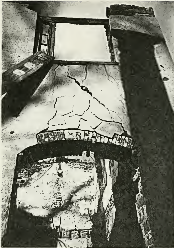
Figure 28: Eastern archway of south elevation showing symmetrical cracking and brick loss
